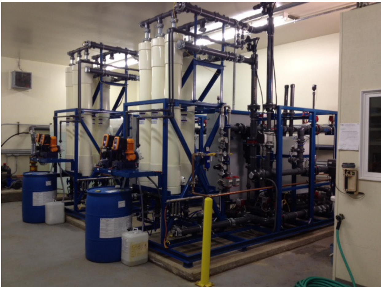
Water Plant Membrane Skids
