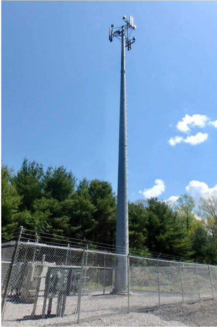
A similar site tower
