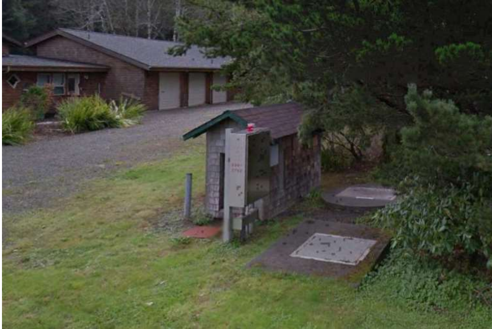
Webb Avenue Pump Station
