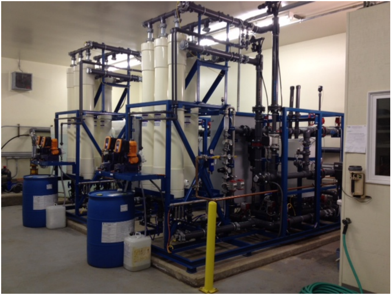
Water Plant Membrane Skids
