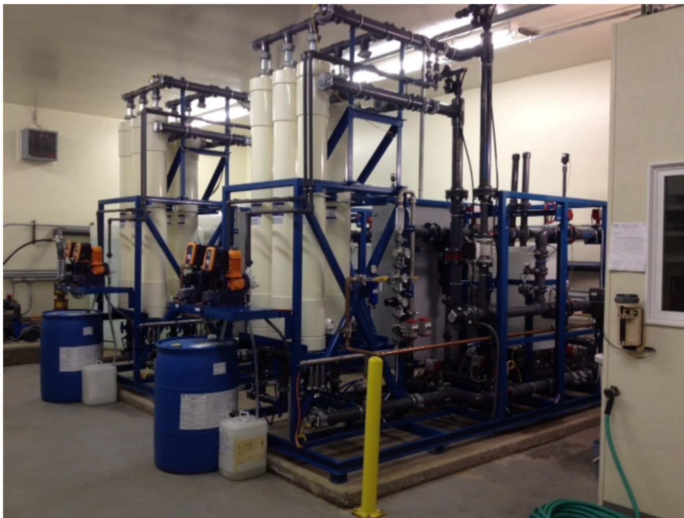
Water Plant Membrane Skids
